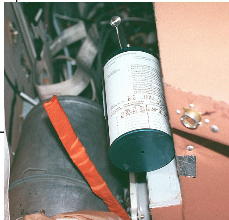
Figure SMP-41 SSAS in Location NM22-190-06
